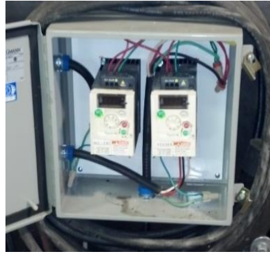
Figure 5.6: Roller and feeder system variable speed drives
