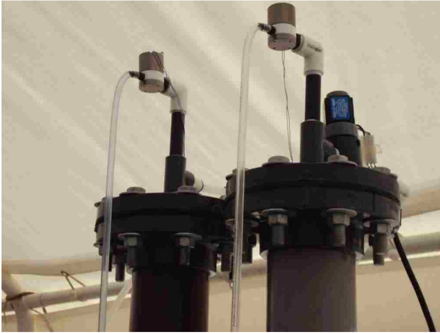
Figure 52: Solenoid Valves at top of Columns
