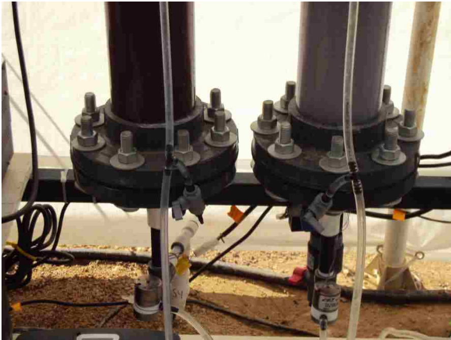
Figure 53: Solenoid Valves at Bottom of Columns
