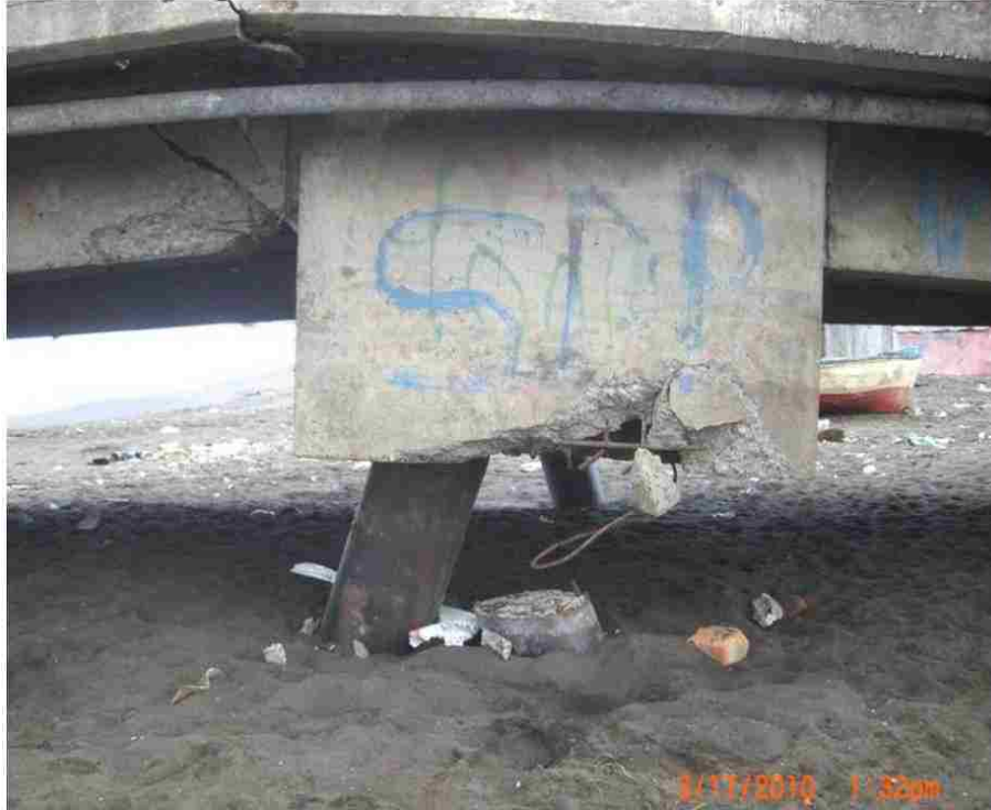
Figure 15. Lo Rojas pier pile cap with battered piles showing pull out of trailing row piles.
