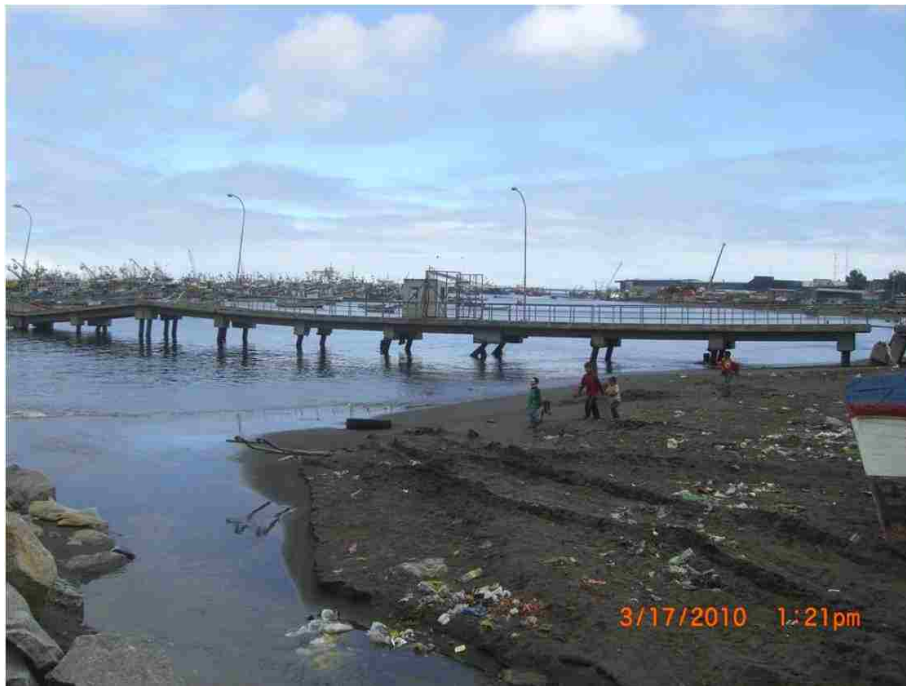
Figure 14. Damages to Lo Rojas pier in Port Coronel due to lateral spreading.
