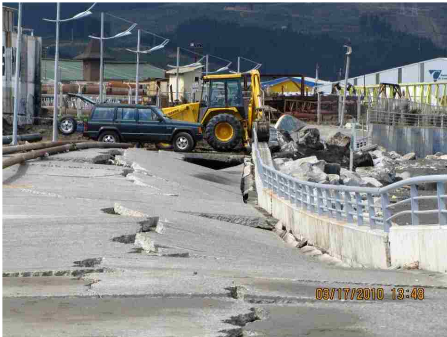
Figure 16. Pavement cracks near Fisherman's (Lo Rojas) pier.
